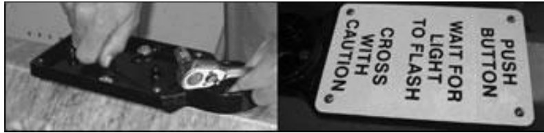
Figure 6-5: Push-button plate (left) and sign (right)
